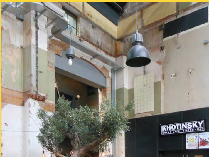
Fig. 5) Detail of the central hall with traces of demolished bathrooms. Energiehuis in Dordrecht, Netherlands. (photo Stefano Francesco Musso 2016)
