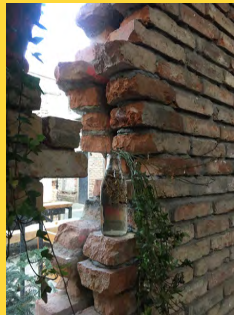
Fig. 7) Acknowledgement of the torn and degraded spaces, partly demolished, providing both aesthetic and "reuse" experience. Vnitroblock, Prague, Czech Republic. (photo Emanuela Sorbo 2019)
