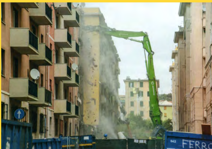
Fig. 2) Demolition of the buildings below Morandi bridge in Genova, Italy. (photo Marco Balastro 2019)
