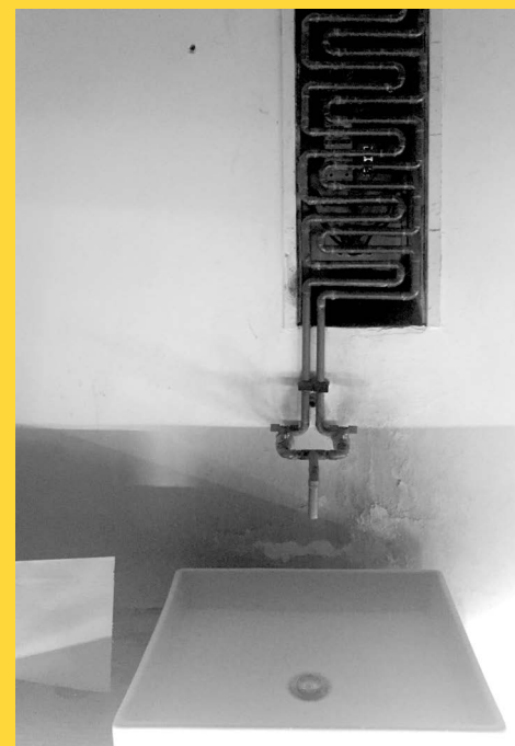
Fig. 13) New water pipe added in full view. Vnitroblok in Holešovice, Prague, Czech Republic. (photo Alessia Zampini 2019)
