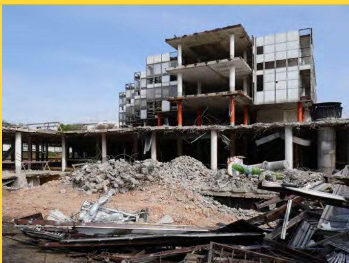
Fig. 6) The Telephone Exchange in Prague-Dejvice during demolition. Czech Republic. (photo Petr Vorlík 2017)
