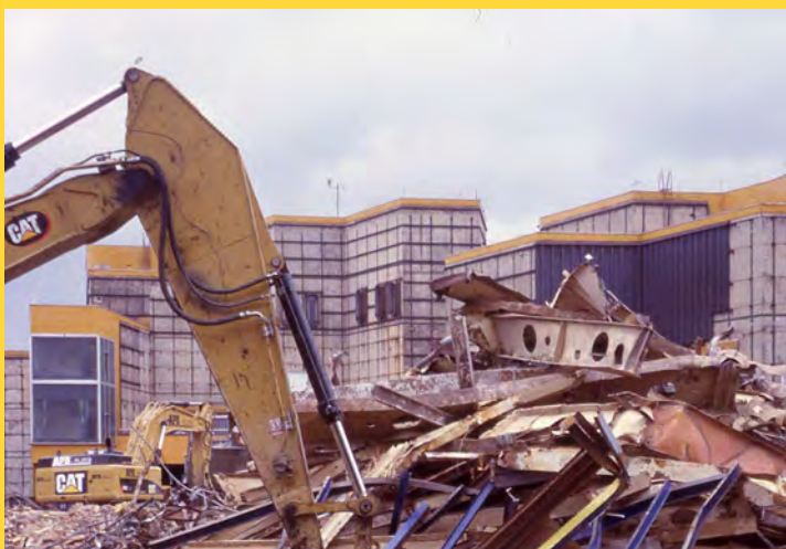
Fig. 2) Demolition of the Ještěd department store in 2009. Liberec, Czech Republic. (private archive of Miroslav Masák)
