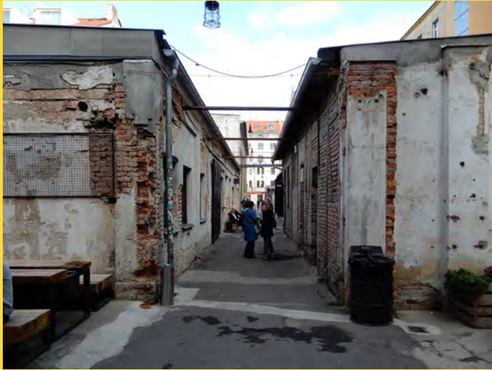
Fig. 1) The internal alley at Vnitroblok in Holešovice, Prague, Czech Republic. (photo Stefano Francesco Musso 2019)
