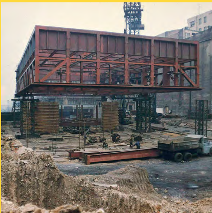
Fig. 2) Administrative and logistic Transgas Complex under construction. Prague, Czech Republic. (private archive of Lucie Loosová)
