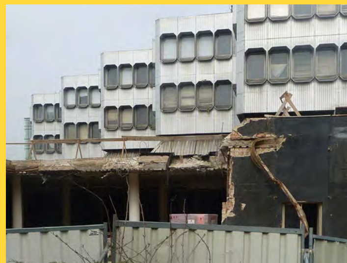
Fig. 4) Telephone exchange stations in Dejvice before demolition. Prague, Czech Republic. (photo Lenka Popelová 2019)
