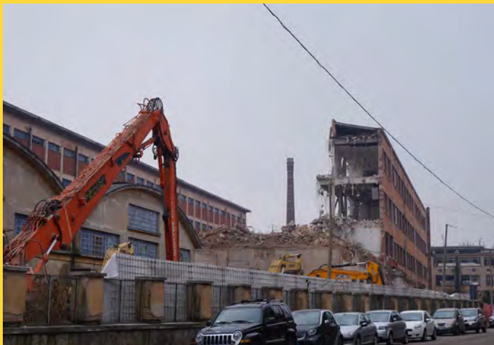
Fig. 7) A building of Tobacco Factory under demolition. Verona, Italy. (photo Sara Rocco 2020)
