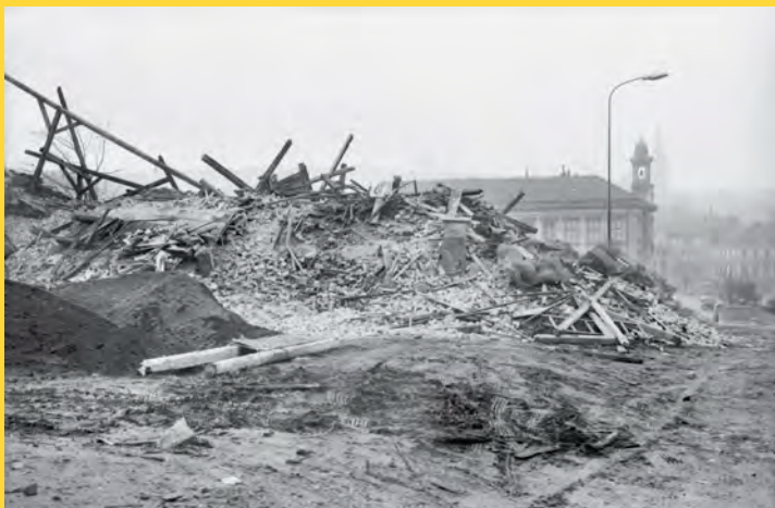
Fig. 1) Demolition of the eastern section of Žižkov. Prague, Czech Republic. (private archive of Ivan Vavřík, photo Jaroslav Kocourek)
