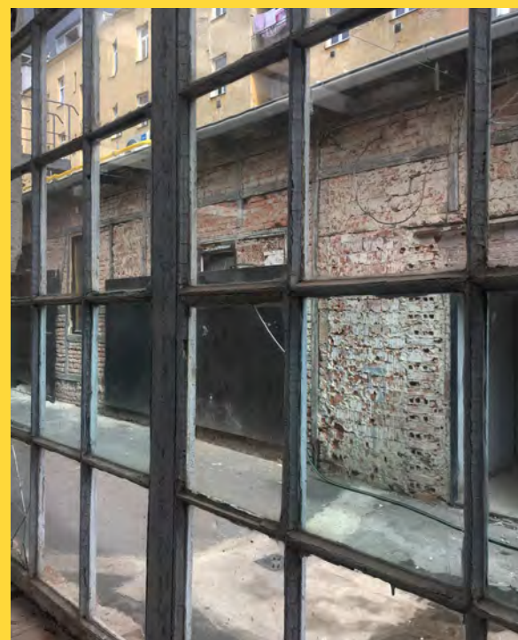
Fig. 6) From the factory's old window in Holešovice, Prague, Czech Republic. (photo Carolina Di Biase 2019)
