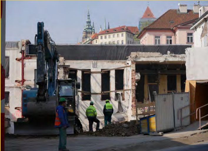
Fig. 9) Demolition of the transformer electrical substation at Klárov in Prague, located very close to Prague Castle. Czech Republic. (photo Petr Vorlík 2019)
