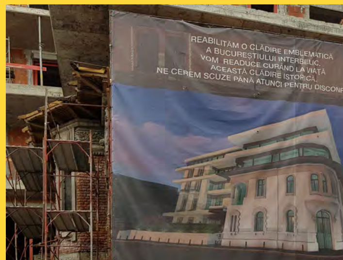
Fig. 10) Façades of the neo-Romanian building embedded in a new housing development. Bucharest, Romania. (photo Rodica Crişan 2019)
