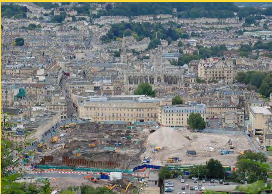
Fig. 4) Demolition of the Georgian Buildings. Bath, UK. ( flickr.com/photos/ sevendipity/1075861033/ sizes/o/in/ photostream/ ), photo Charles Stirton)
